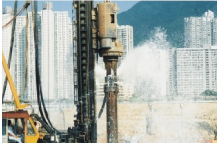
Foundation Foundational construction of buildings and bridges up to 32''(Ø800) of casing diameter.
