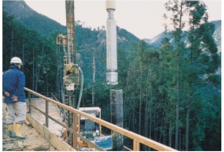
Piling After casing through the collapsing overburden, insert a H-steel, then pull up the casing.
